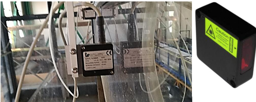
Figure 17: Laser sensor installed (model LCL45/100 U-485 BI5M).
