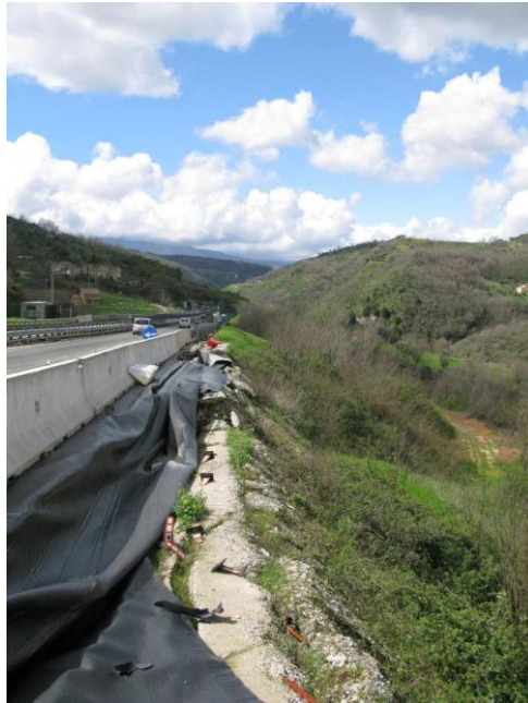
Figure 39. A3: Edge break in the Mancarelli site
