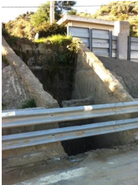
Figure 43. A18: gate conveying mudflow over roadway
