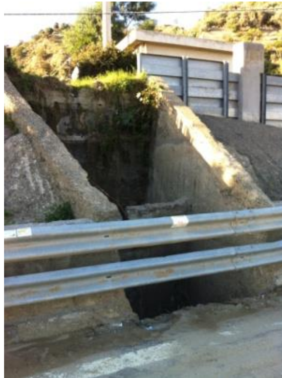
Figure 42. A18: gate conveying mudflow over roadway
